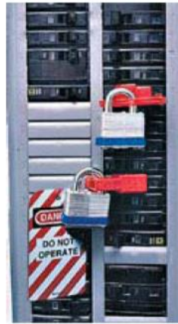
Danger tagged circuit breaker locking off devices
